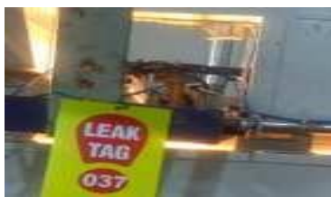
FLOW CONTROL VALVE
