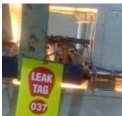
FLOW CONTROL VALVE
